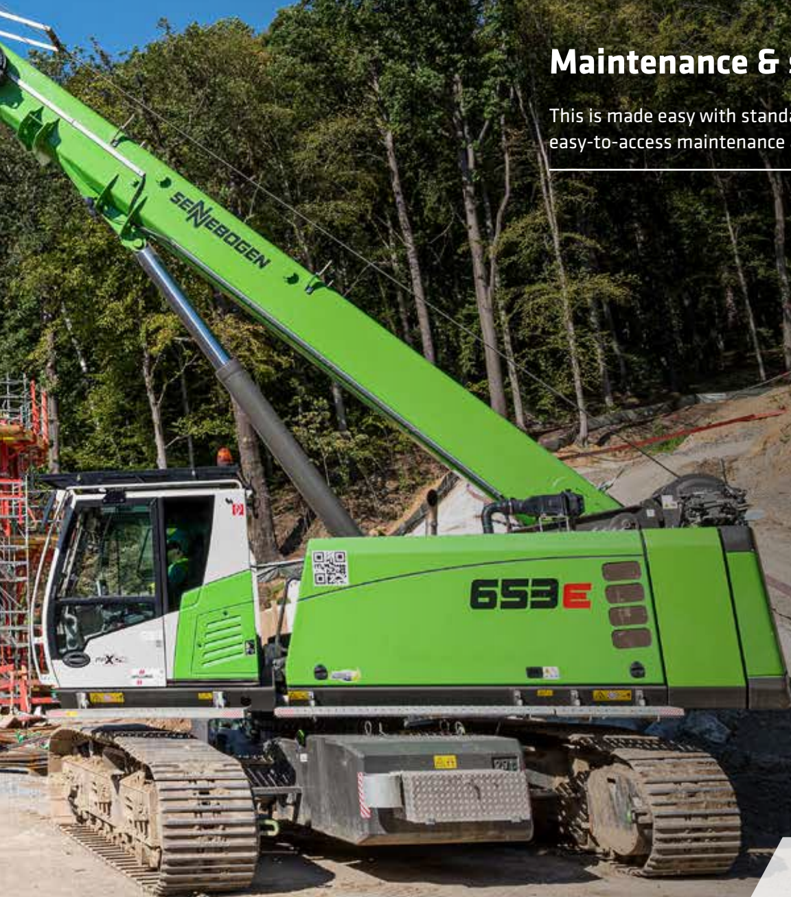
The photo shows the 653 E with 13 m fly jib in bridge construction, Germany.
